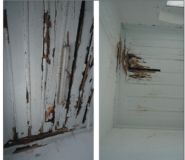
Figure 22. Swelling and material decay caused by water from the roof, especially on the ceilings of the upper floor spaces
