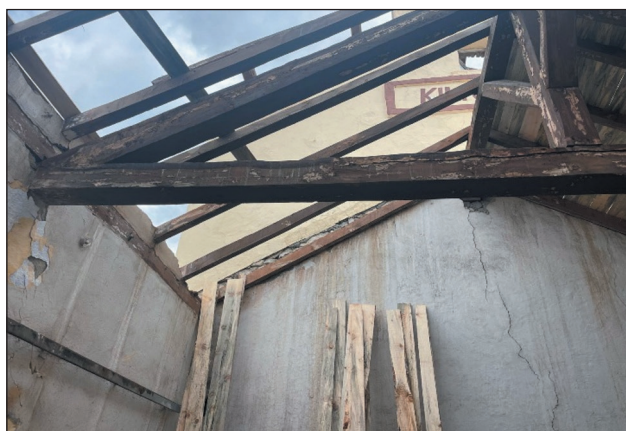
Figure 8. Condition of the roof before simple repair
